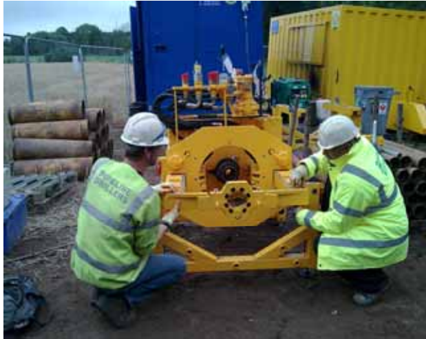
Pipeline Drillers engineers preparing the Perforator ® PBA85 V pilot bore/HDD system on site.
