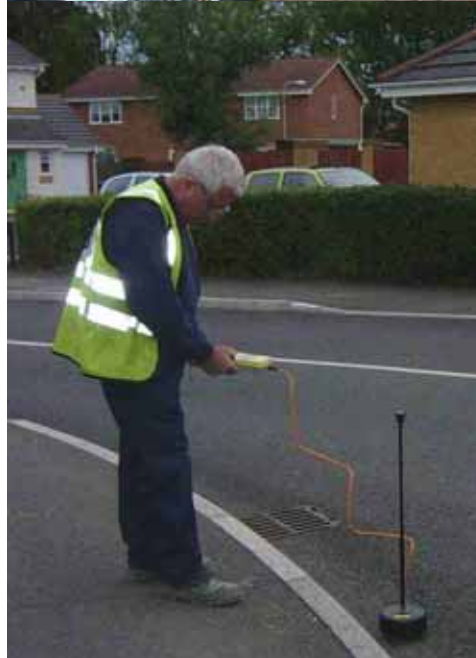
The Gas Tracker system - The signal generator attached to the meter box (above) and tracking the pipeline route (below).
