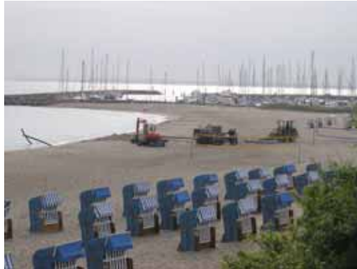
The Grundodrill 15N being driven to the starting point on the beach.
