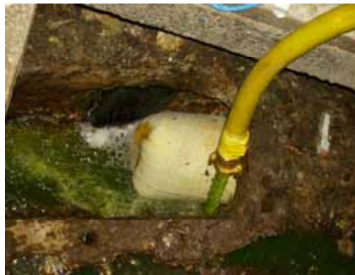
The inverted liner reaches the reception manhole and is ready for curing.
