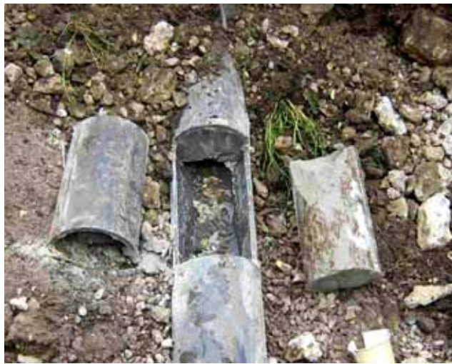
The rising main opened for access shows just how restricted the pipes were by the wax.
